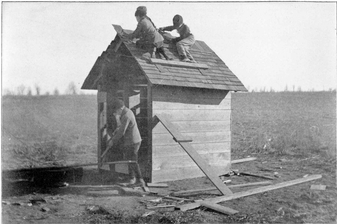
HOUSE BUILT BY THIRD AND FOURTH GRADES. (By Permission of Miss Eleanor Phillips.)
